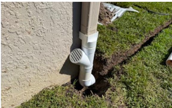
PVC connection on gutter by pool equipment
